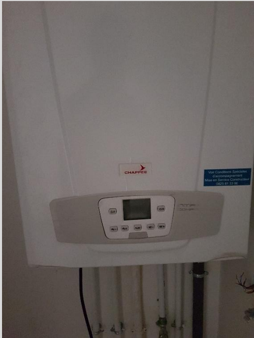
Chaudière gaz individuelle (ECS + chauffage)
