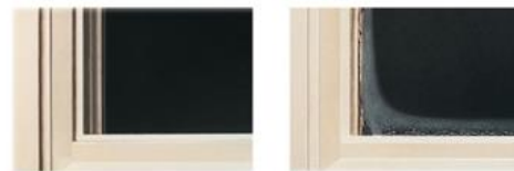
Condensation and window edge.
