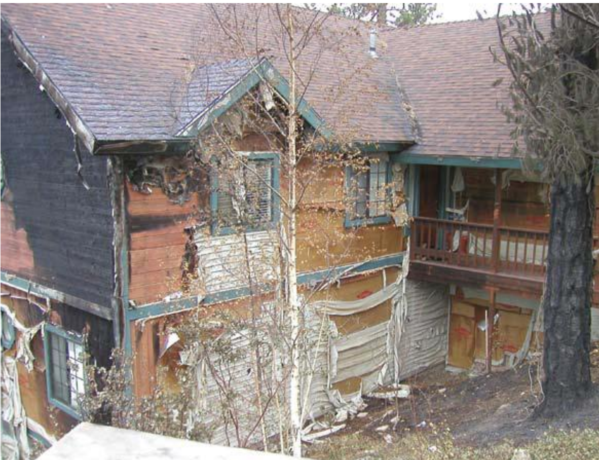
Figure 32. Home at 26150 Walnut Hills Dr. Thermal exposure from the destroyed home at 26142 contributed to the vinyl sloughing off. Surface fire burned the vinyl siding and under-layment on the northwest side (left) and worked its way up the wall burning the wood siding. Blackened asphalt shingles in the roof valley (center top) are from accumulated needles that burned.
